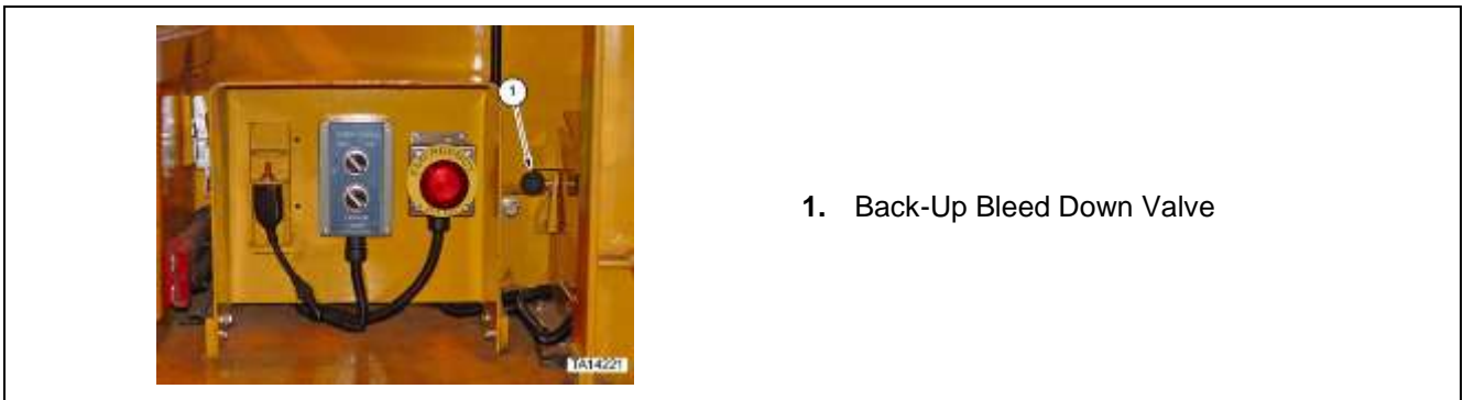
Figure 44. Back-up bleed down valve (ground location access)
