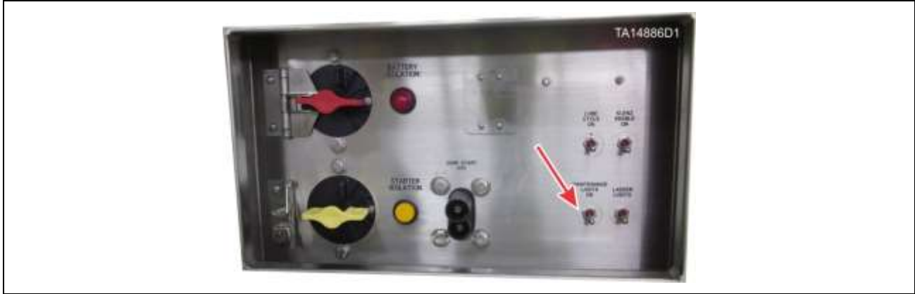
Figure 31. Maintenance lights switch
