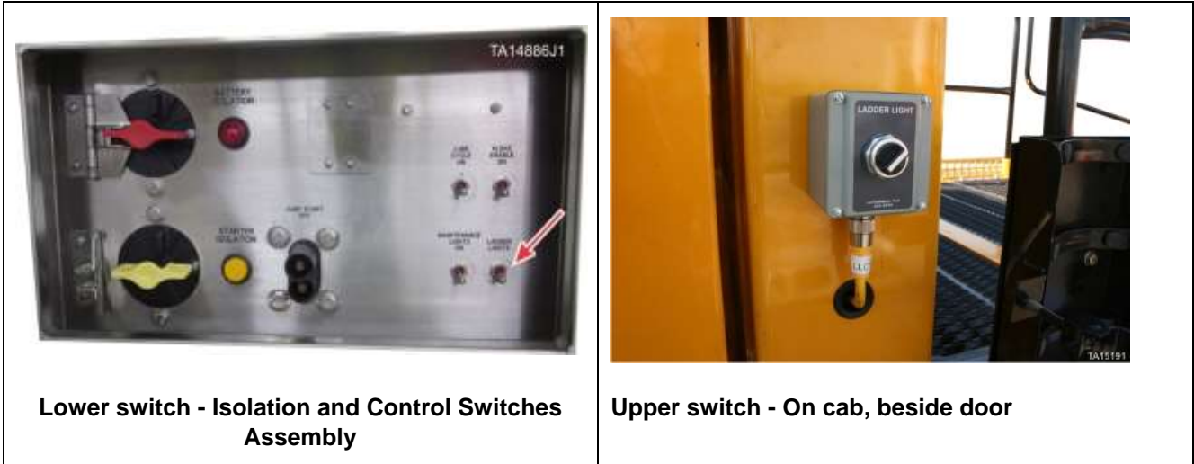
Figure 30. Ladder light switches
